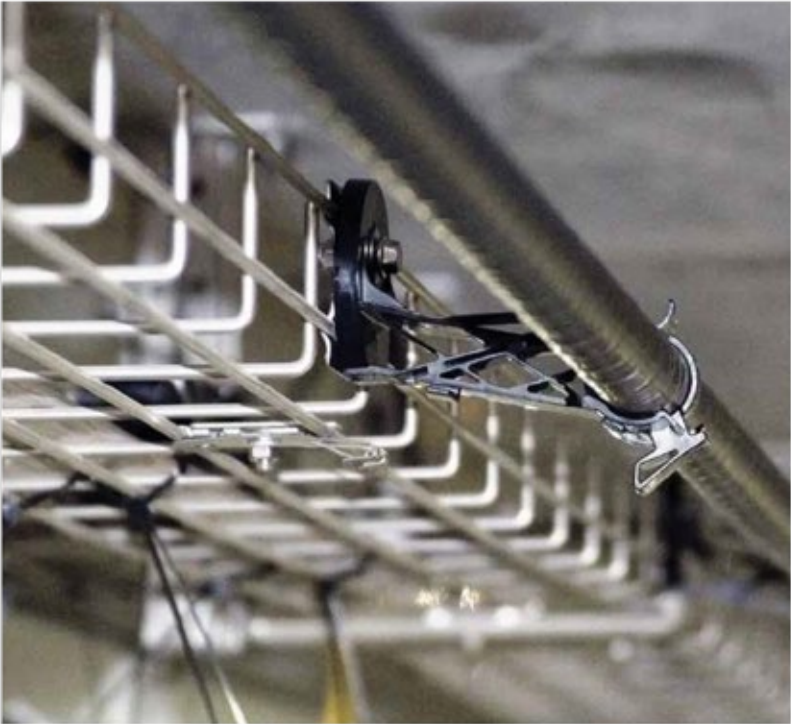
The radiating cable is mounted on a mesh track in a tunnel using CLIC SKH.
